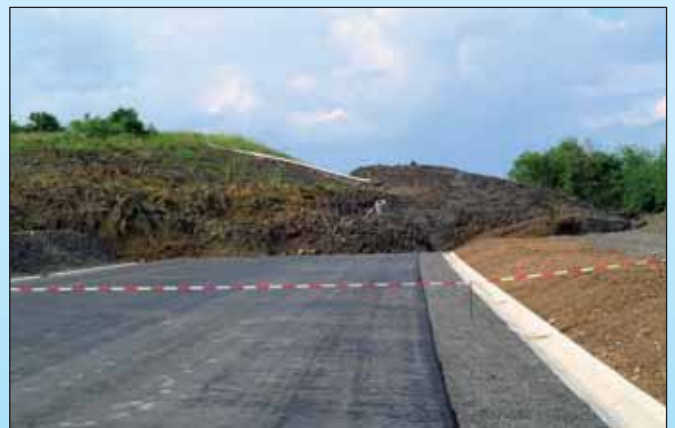
Fig. 5.7 Landslide Accumulation on D8 Motorway Body (Source: ČGS).
